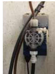
Iron system – be careful in trusting this alone!!!
